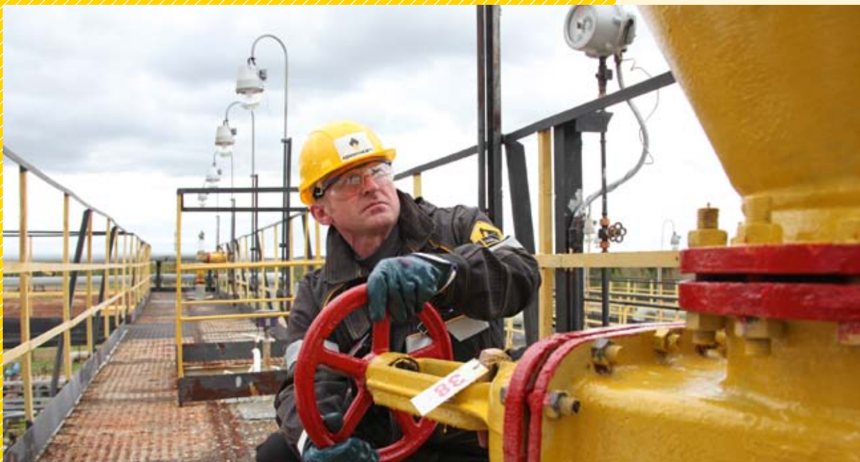
Udmurtneft, operator of a dewatering and desalting unit Alexei Zamaraev
